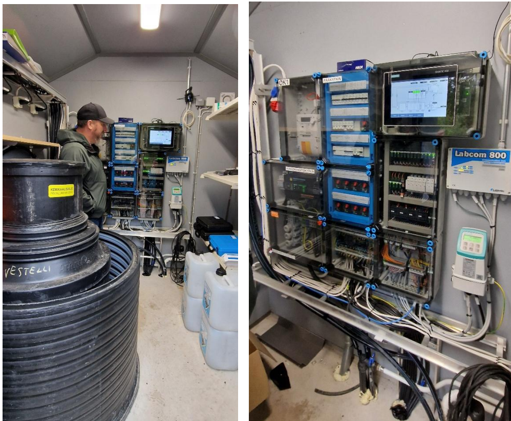
Picture 7. Johan Holmberg, Managing Director of the Barösund Water Cooperative, is responsible for managing the wastewater treatment plant. During the summer, he gained practical experience in operating the Labcom 800 system and monitoring its performance.
