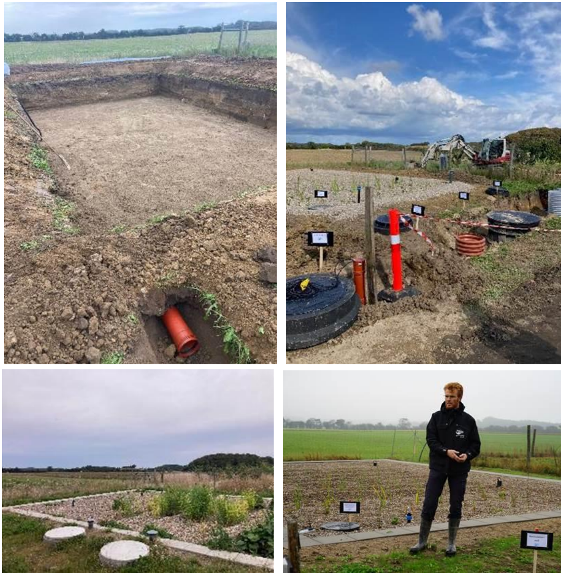
Figure 14. Pictures of the plant during and after construction in 2023. (Picture: Danmarks Naturfond)
