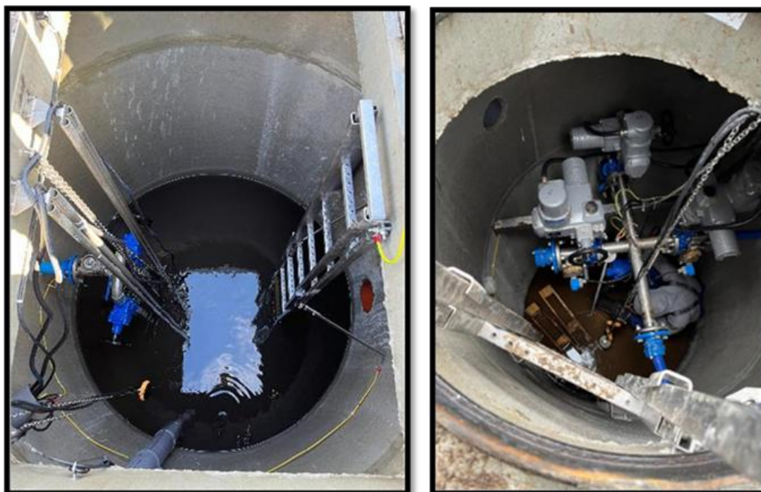
Figure 24. Pumping station P3 (left) and collection well (right) at the Bure Misie Settlement wastewater treatment plant. (photos: Płuciennik M., BMCF)
