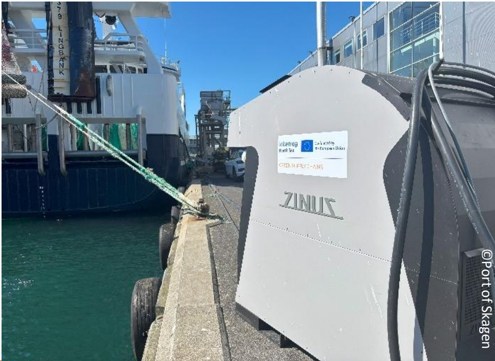
Cable Management System (CMS) at the quay
