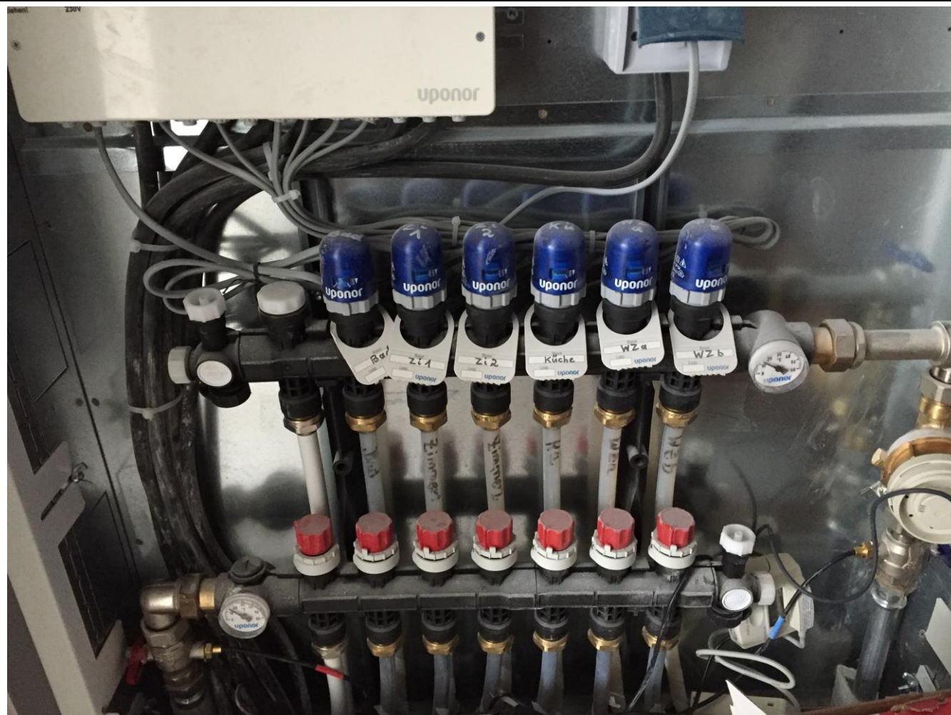
Figure 12: Pre adjustment of floor heating system © ZEBAU
