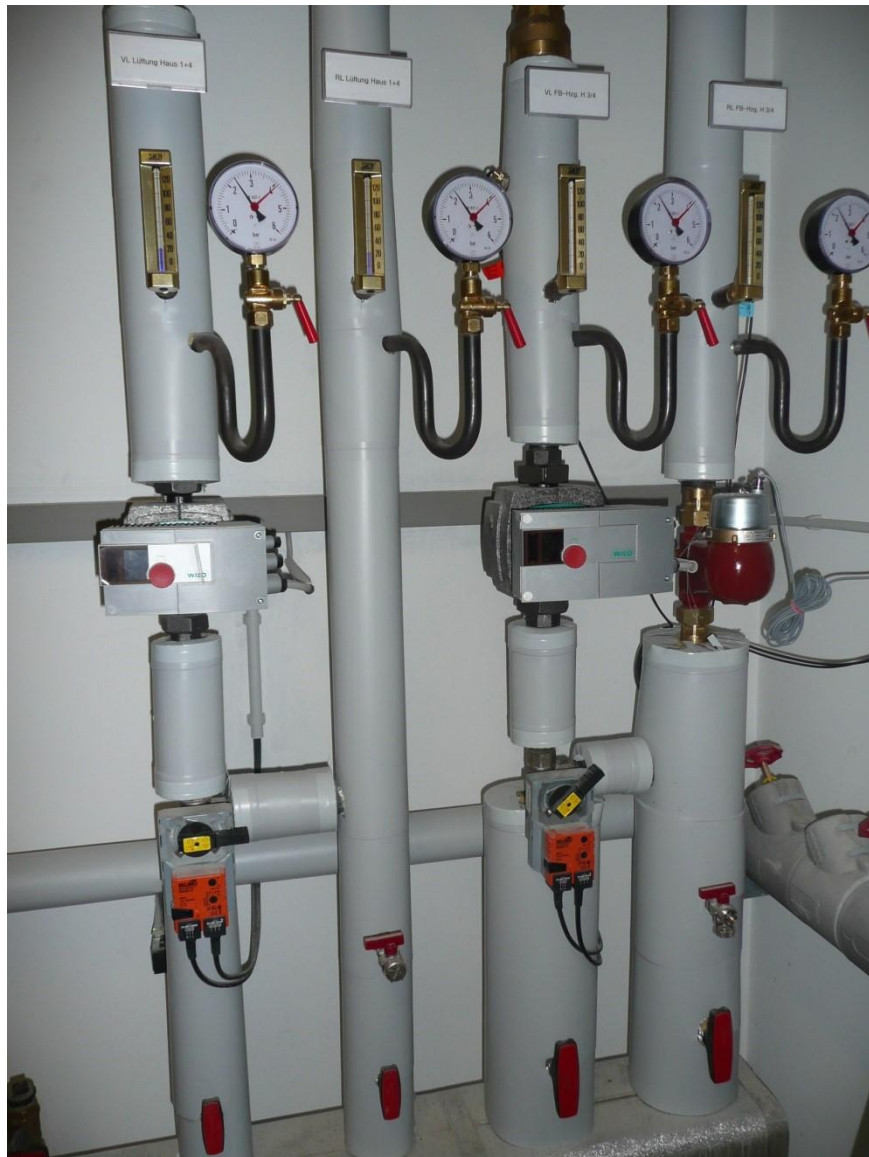
Figure 11: Insulated heating pipes © ZEBAU GmbH
