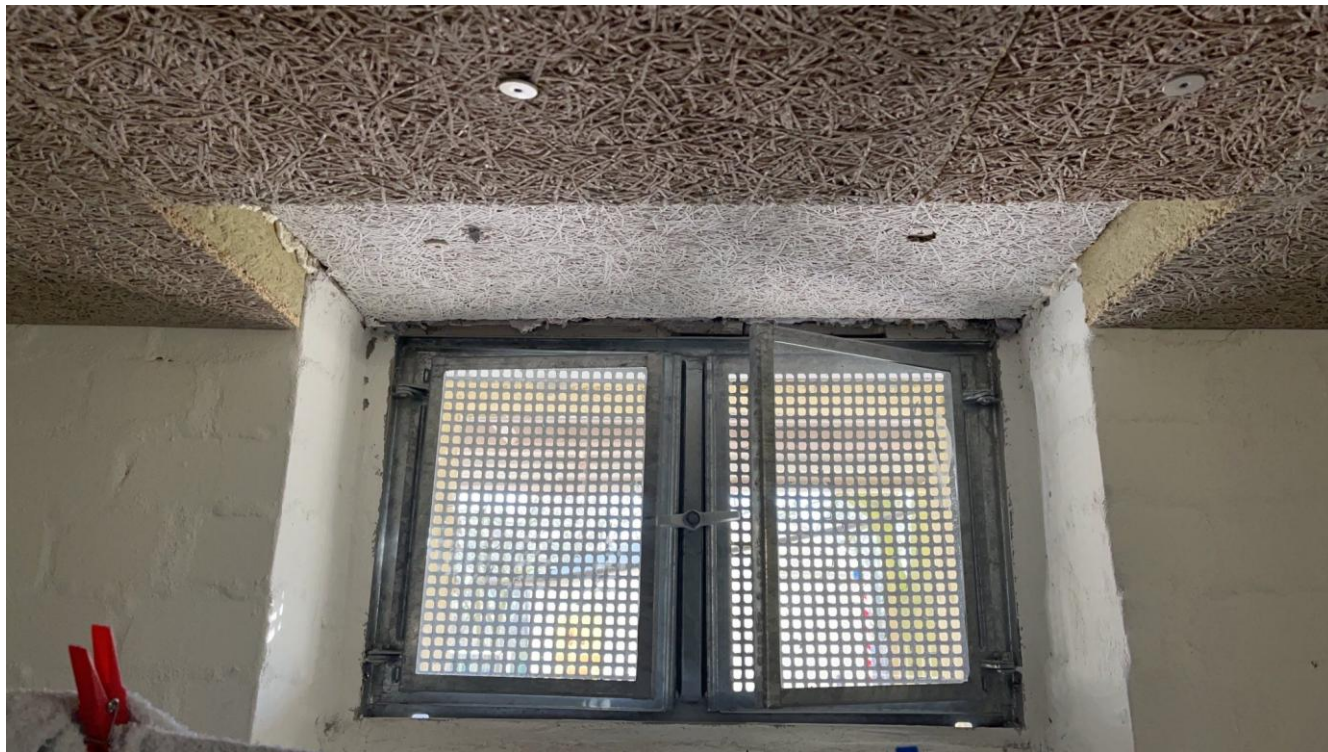
Figure 2: insulated basement ceiling © ZEBAU GmbH
