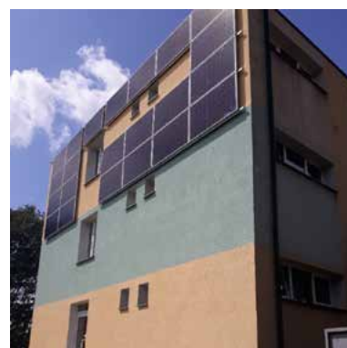
Public utility building installation supporting the system in Turośń Kościelna
