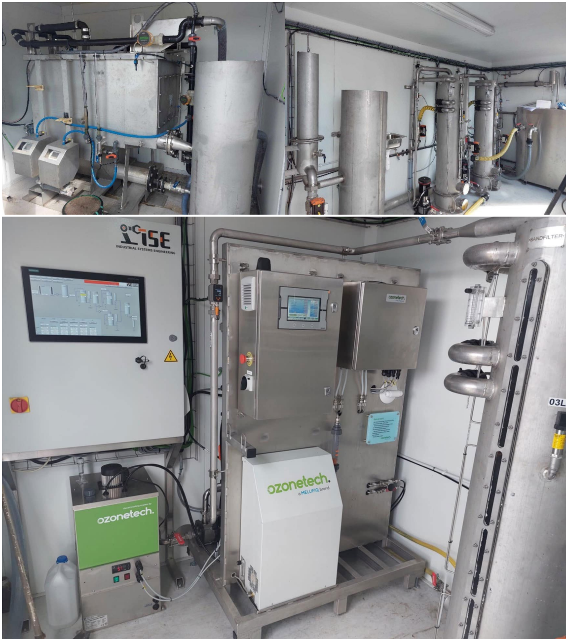
Figure 2. View of the pilot plant interior
