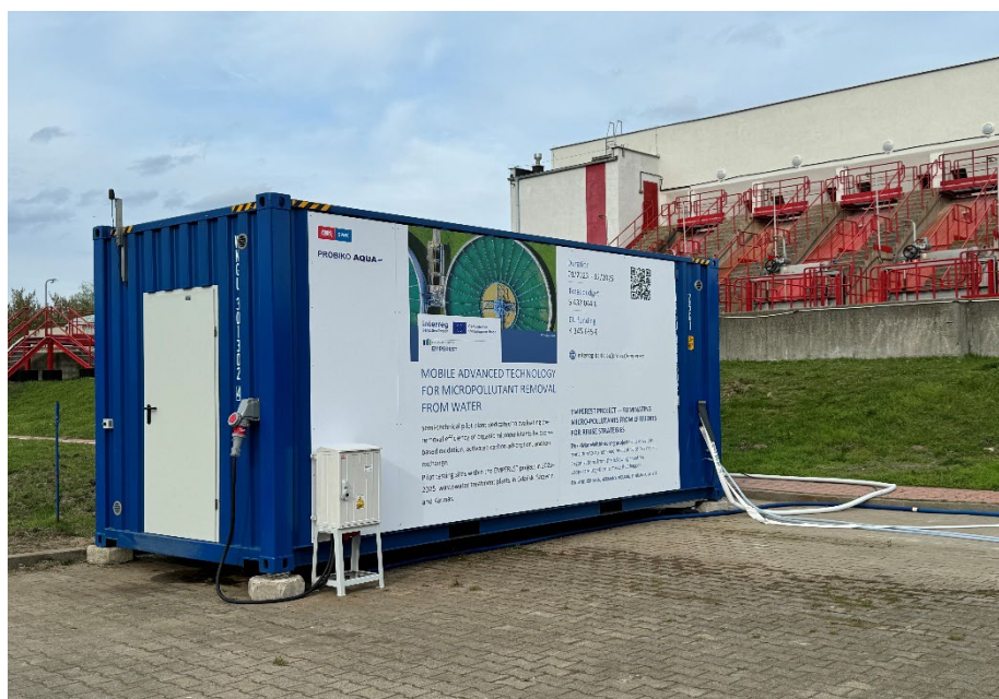
Figure 1. View of the pilot plant located at the Wschód WWTP in Gdańsk.
