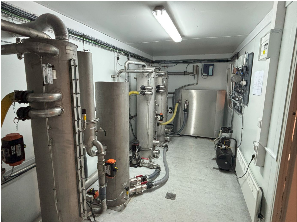
Figure 2: View of the pilot plant interior
