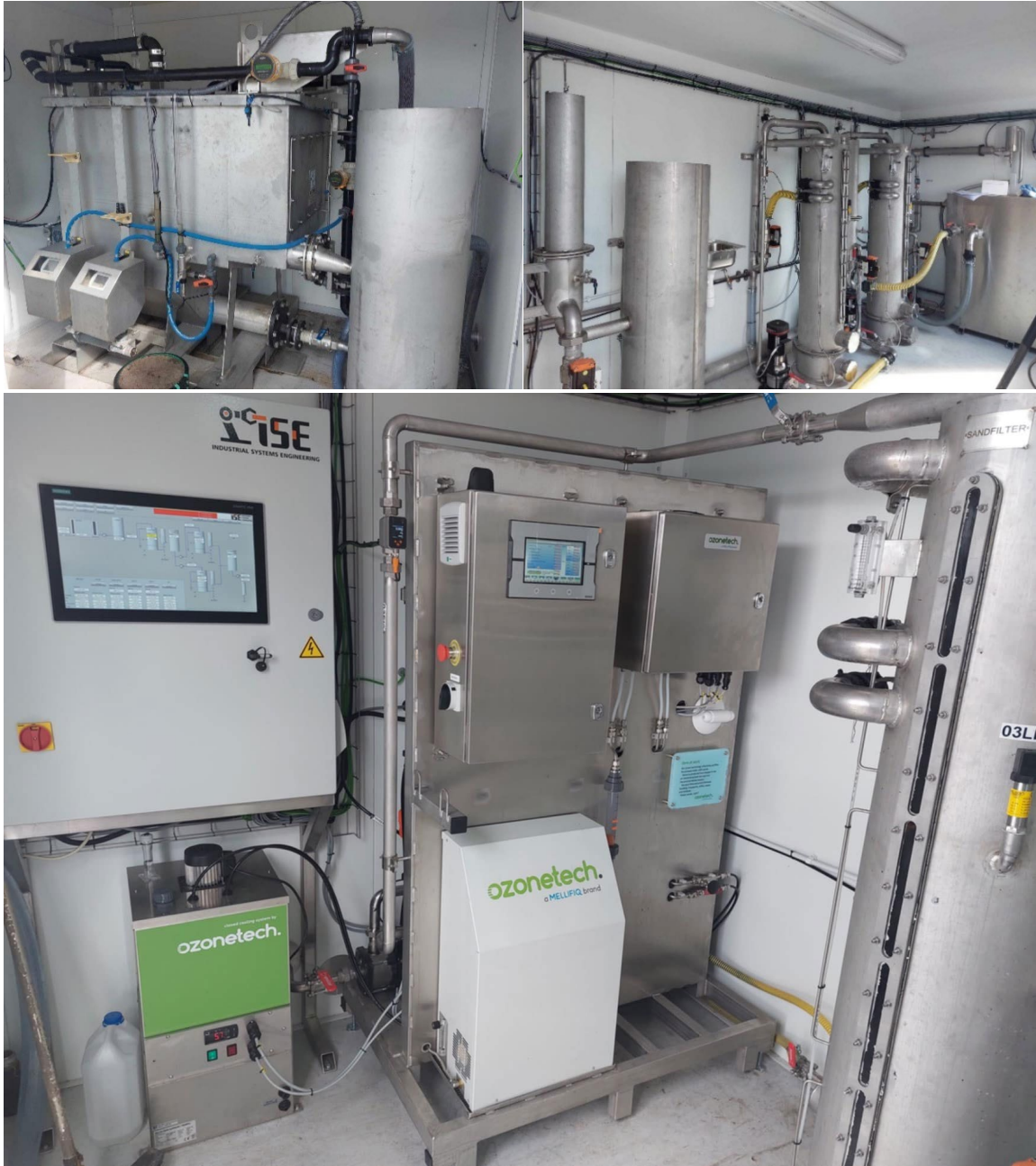
Figure 3. View of the pilot plant interior
