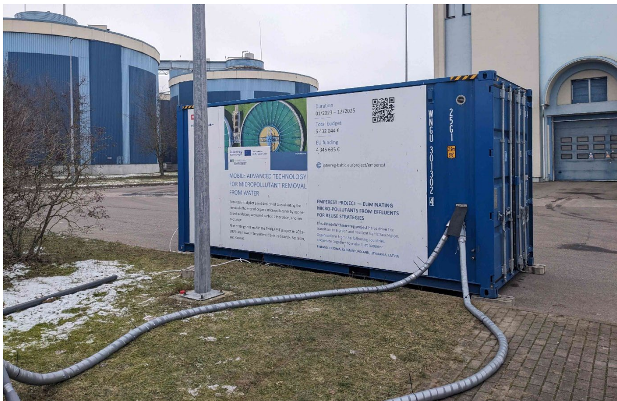
Figure 1. View of the pilot plant located at the Kaunas WWTP.
