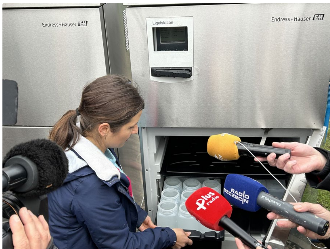
Figure 7. Two of four automated sampling stations at WWTP Pomorzany in Szczecin.
