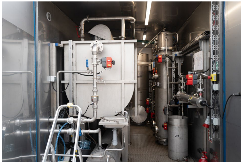
Figure 2. View of the pilot plant interior.
