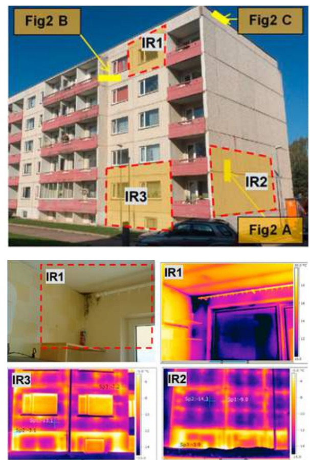
Figure 2. Overview of the pilot building (dormitory) before renovation from the outside (left) and in thermal camera images (right). Source: Pihelo, P., Kalamees, T., & Kuusk, K. (2017), “nZEB Renovation with Prefabricated Modular Panels”, in: Energy Procedia (vol. 132, pp. 1006–1011). Elsevier BV. https://doi.org/10.1016/j.egypro.2017.09.708
