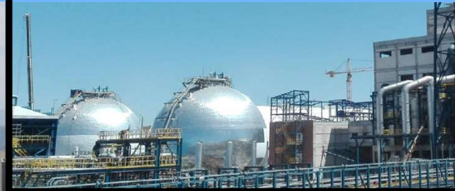
ETIR BAKIR, Mazidagly, Turkey Ammonia Storage Facility incl. 2 x 5,480 m 3 Tanks
