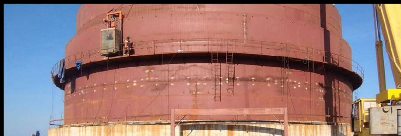
Eti Bakir A.S., Turkey Anhydrous Ammonia Terminal incl. 1 x 15,000 MT Storage Tank
