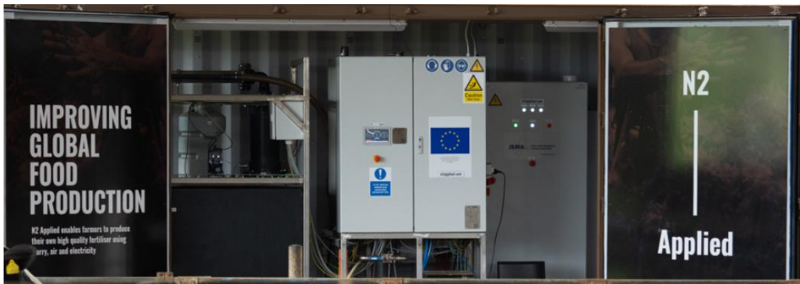
Figure 10: N 2 -applied unit – pilot plant container (N 2 APPLIED)
