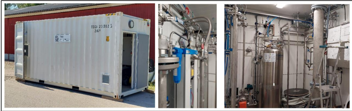
Figure 13: Container unit CO 2 -Liquefaction plant TB12 (RISE)
