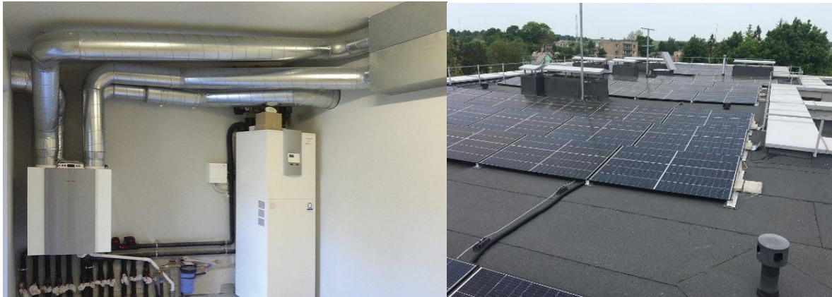
Fig. 3. Heat pump in the building and PV on the roof of the building
